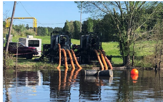
Exhibit 1 Surface Water Pumps on Lake Bistineau March 2020
